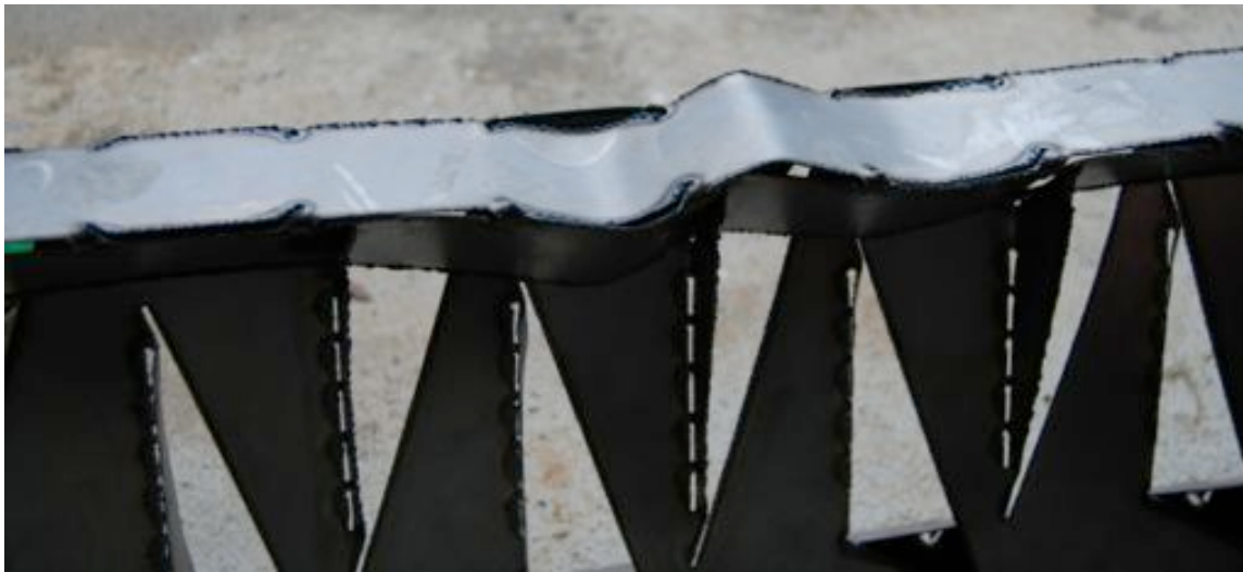
Figure 3. Localized failure of the top chord of bi-chord truss
